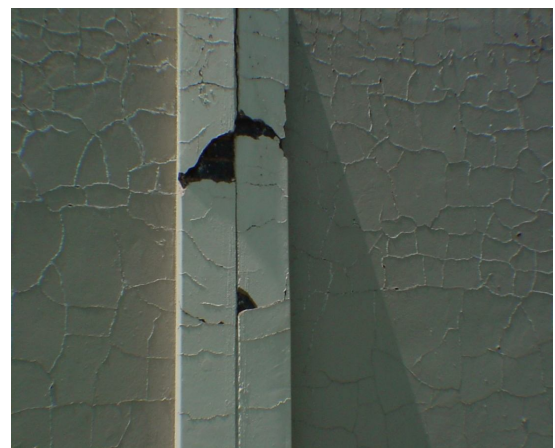
Photo DSC01139. An inadequately water-proofed, plastered wall built with clinker bricks, which contained undue amounts of sulphate. Note the excessive crazing and the efflorescence in and paint failure along the cracks as well as spalling of plaster from a column due to expansion of the brickwork.
