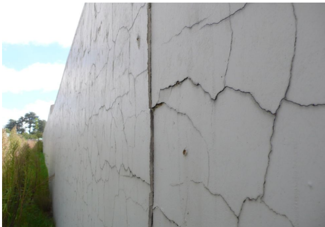
Photo 1000984. Cracking and adhesion failure of plaster next to a movement joint in an inadequately water-proofed, exposed wall, caused by expanding clinker brickwork containing excessive amounts of sulphate
